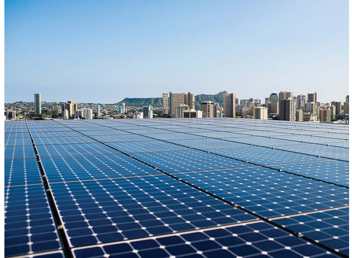
Solar Panels on the roof of the Kapiolani Medical Center parking garage on the island of O‘ahu. While the number of jobs in Clean Energy and Energy Efficiency has increased on all islands, O‘ahu now has 75% of the state’s jobs in these two core areas. Image source: Earthjustice.org
